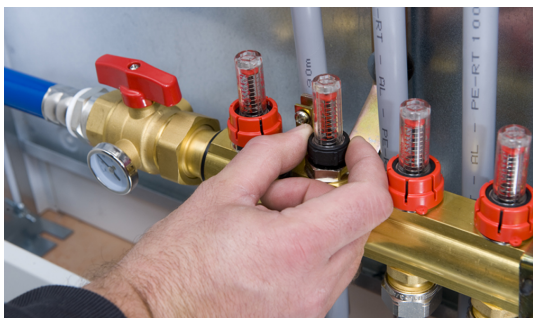
Fig. 7: Open ball valves and all flow meters completely.
